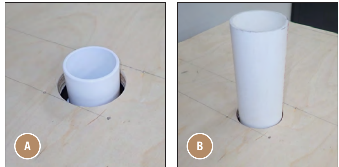
FIG. 5. Cut the coupling (A) and the PVC tubing (B) flush with the countertop.
