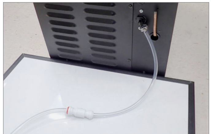
FIG. 5. Installed check valve.
